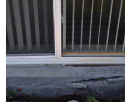
Cracking at Windows
